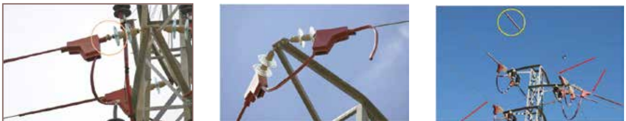
Figure 11: Examples of covers that were not placed properly leading to partial or complete exposure of the energized parts. A) Exposed live metal part ©Justo Martín. B) Poor fitting of conductor cover leading to detachment ©Justo Martín. C) Poor fitting of conductor cover leading to detachment and movement along the conductor ©James Dwyer. (source: Martín Martín et al., 2022).
