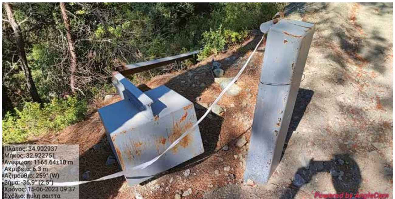
Figure 4: Saitta case, the gate was destroyed as a result of a vehicle strike. Possibly the stakes were moved. With the re-installation of the new barrier, there may be problems in closing the gate. Michael Zacharias©Forestry Department Archive.
